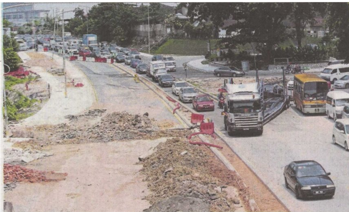
Traffic has been reduced to a crawl in Jalan Utara, Petaling Jaya, due to road repairs. Pic by Ghazali Kori
